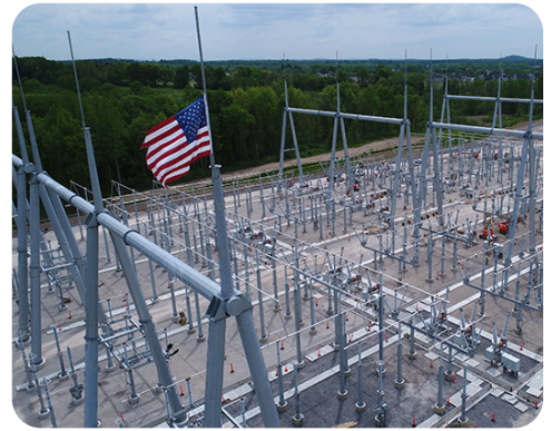
Construction of the new Station 255 in the Town of Henrietta, above, is part of the Rochester Area Reliability Project.
