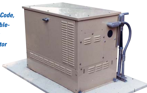
Typical stationary natural-gas fired generator
